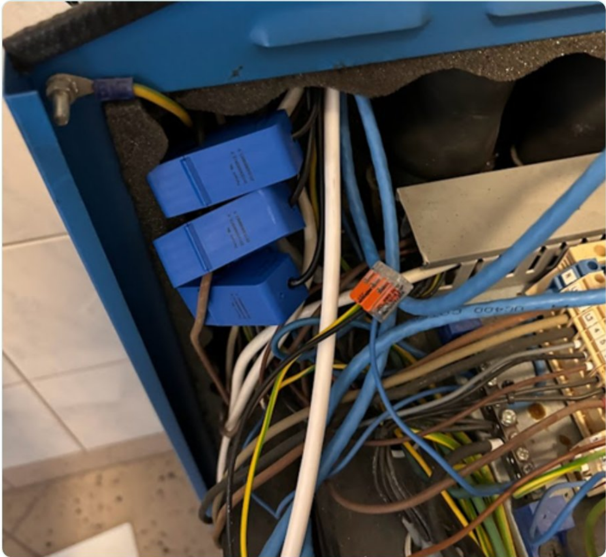
Current sensors on the phase wires
