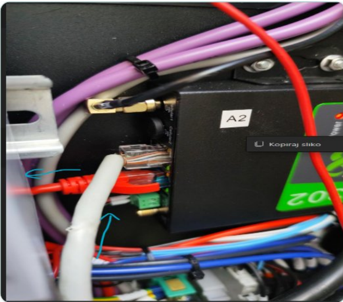
White cable to the top ETH port of the router
