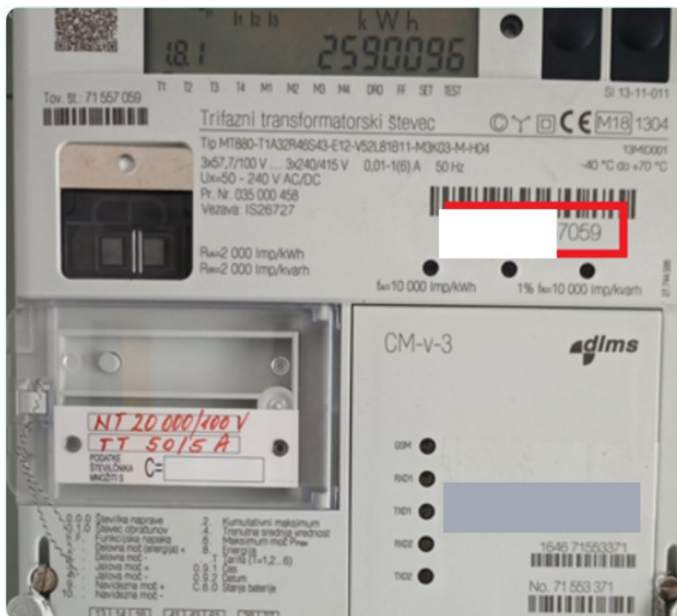
Serial number on the energy meter
