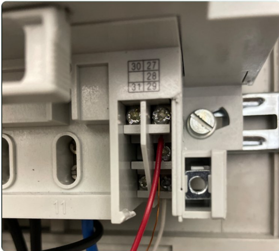
Terminal block on the energy meter
