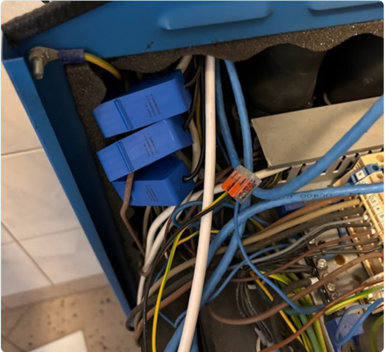
Current sensors on the phase wires
