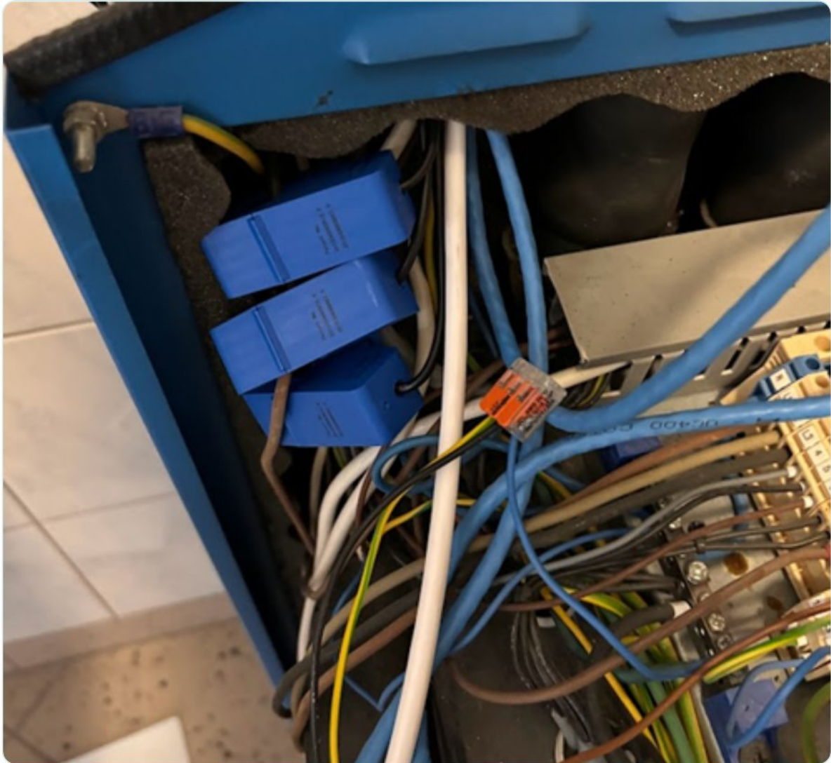
Current sensors on the phase wires of the heat pump
