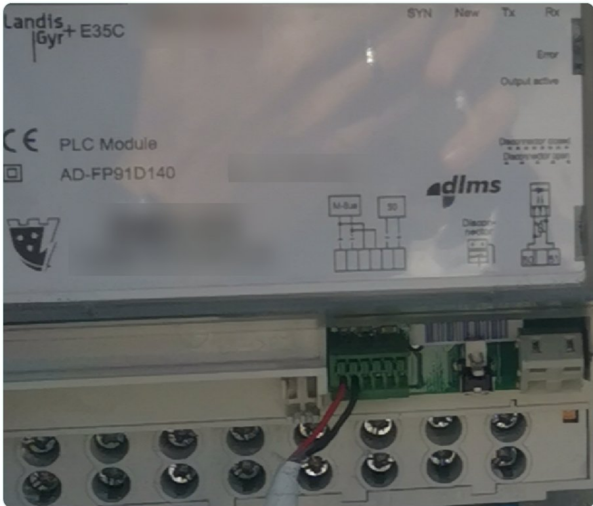
M-Bus pins on the energy meter
