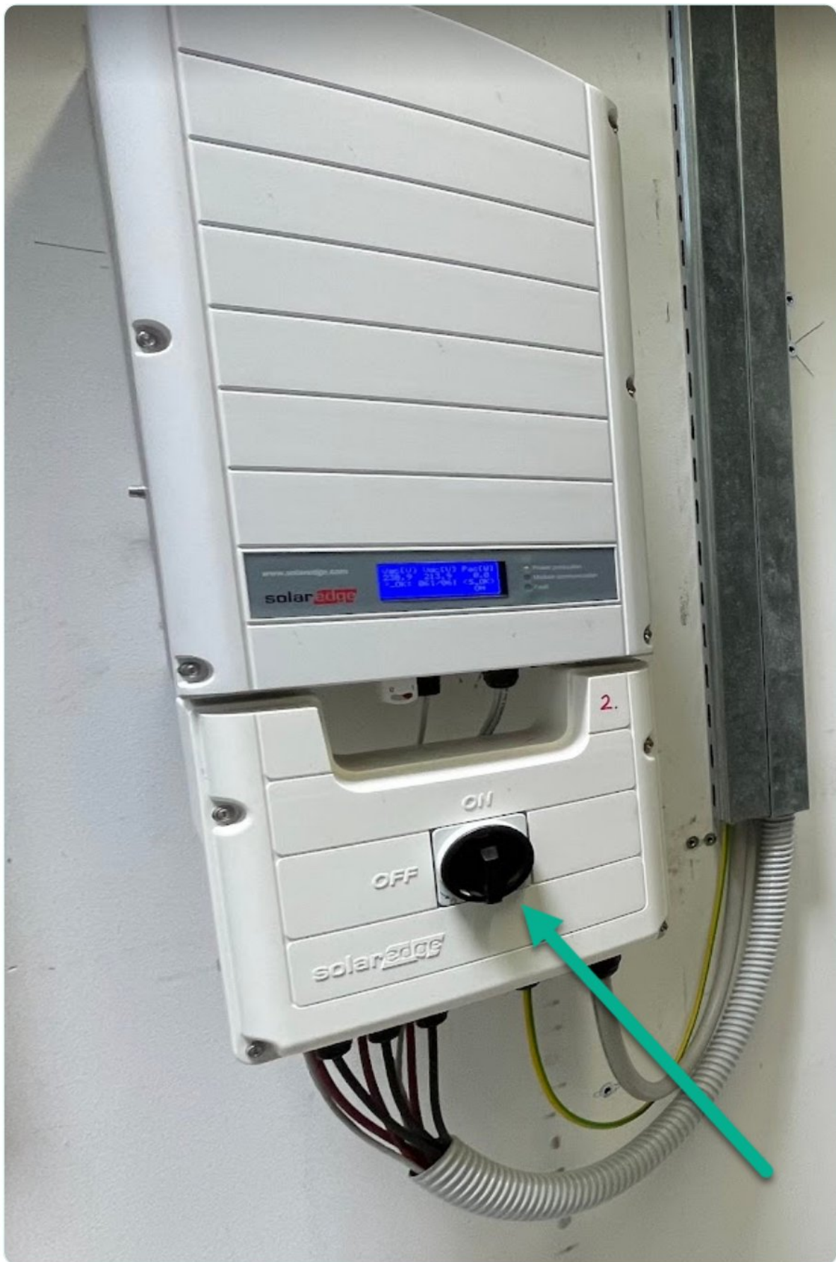
Main switch in the OFF position
