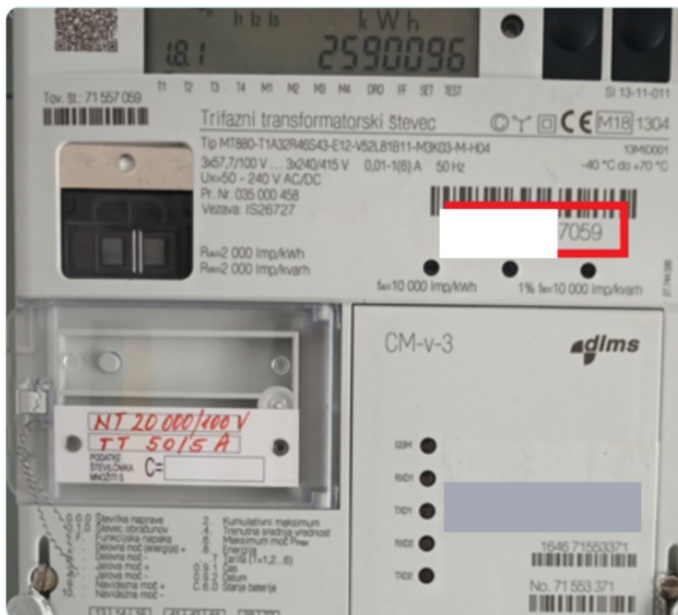
Serial number on the energy meter
