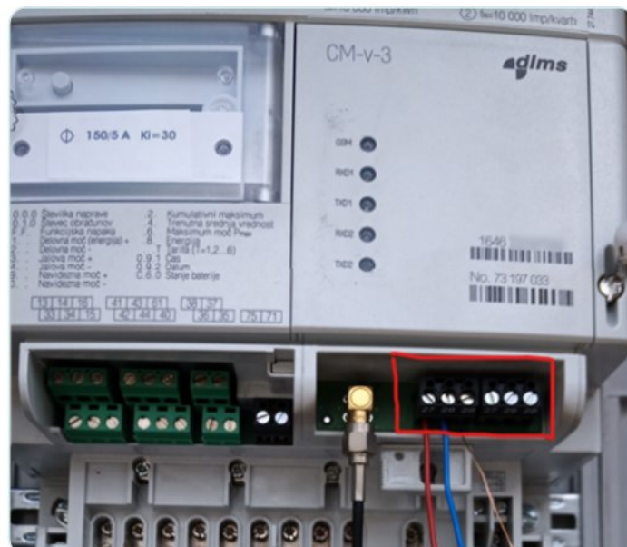
Energy meter with the CM-v-3 module
