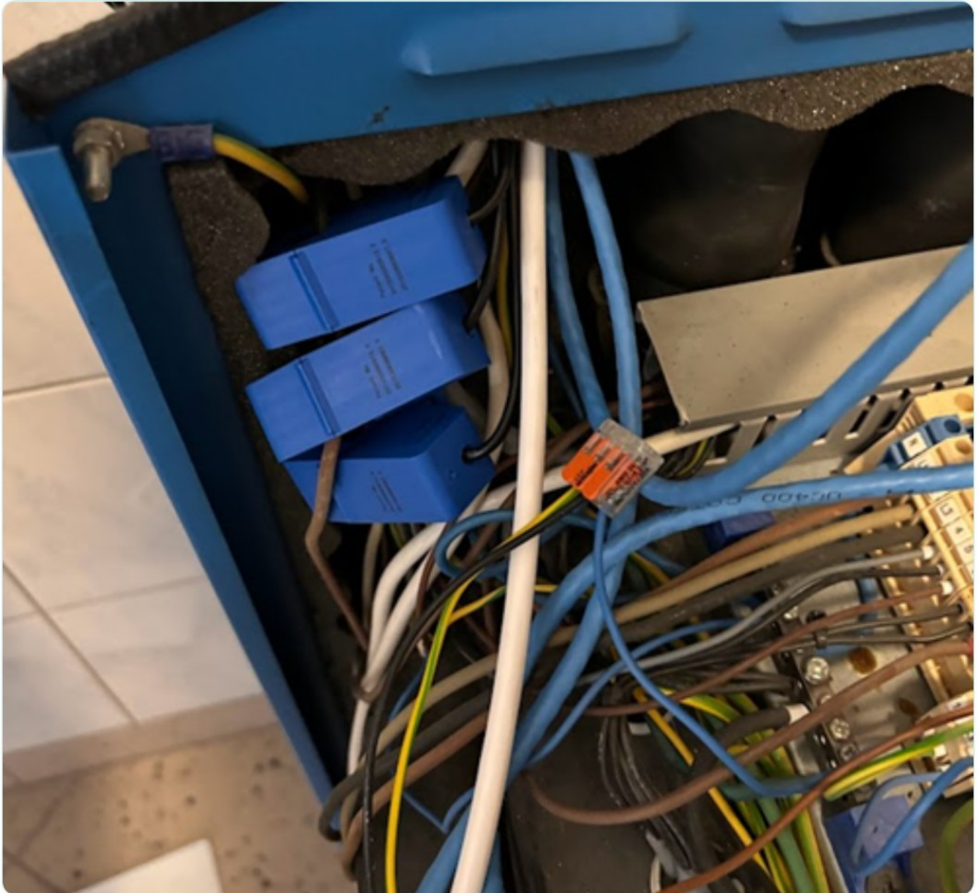
Current sensors on the phase wires
